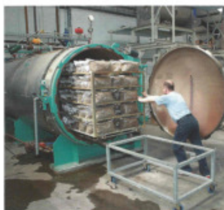
At the autoclave in the new building.
